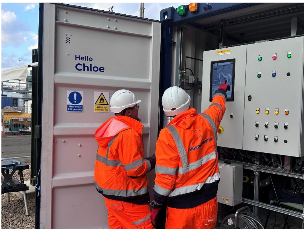
Figure 4. Control panel of Chloe outside at the entrance of the shipping container
