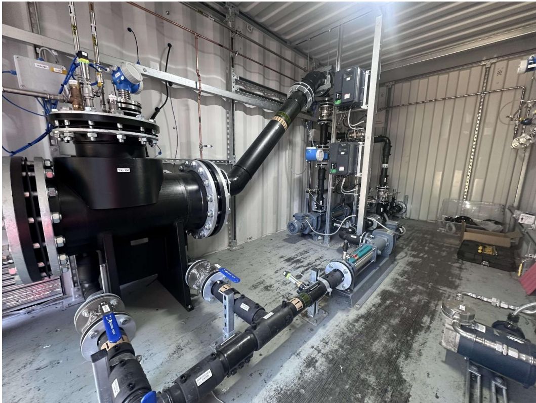
Figure 3. Photo of Chloe installed inside a shipping container
